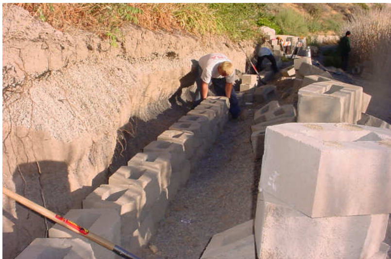
The Lake Trail wall that collapsed last spring is being repaired. Thanks to funding assistance from SSD and SSOA.
